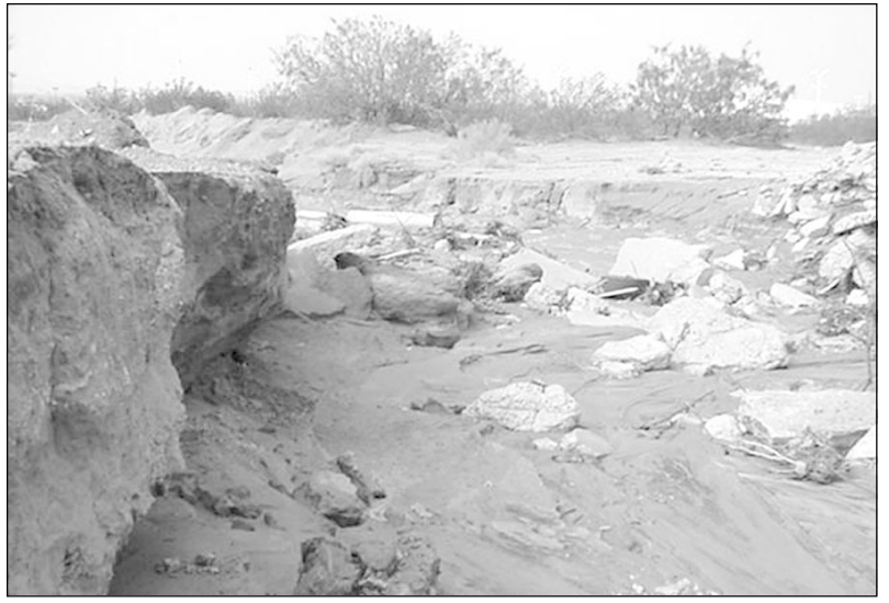
GONE WITH THE WATER — Erosion in water courses is a constant problem in the East County, even through El Paso has little rainfall. In this ravine, an attempt has been made to slow erosion by depositing chunks of broken curbs and busted asphalt from other locations.
