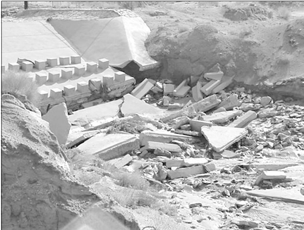
BUILT ON SAND — Even with state-of-the-art erosion and flood control built into major waterways, the elusive "sugar sand" that covers the El Paso landscape melts away beneath, causing portions of the structure to collapse.
