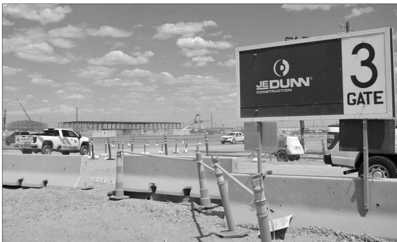
IN AND OUT – This is one of several gates giving workers and deliveries access to the building site.
